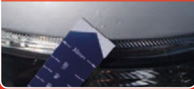
Poor repair: paint blisters around lamp
