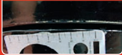
Discoloured panel: rear door not fitted to acceptable standard
